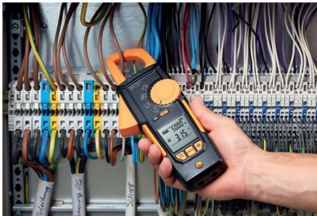
Measuring current in a switching cabinet.
