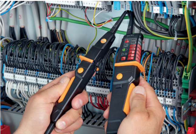
Measuring voltage in a switching cabinet.
