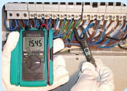
Measuring current in a Switchboard
