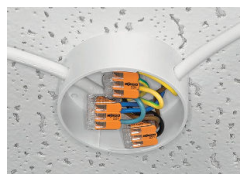
Lighting distribution in a ceiling canopy
